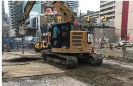
Fig 6: Example of well-prepared working platform that incorporates the use of steel plates to spread the load
