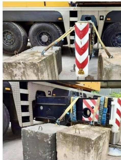
Photographs show concrete blocks and slings being used to hold down an extended crane outrigger
