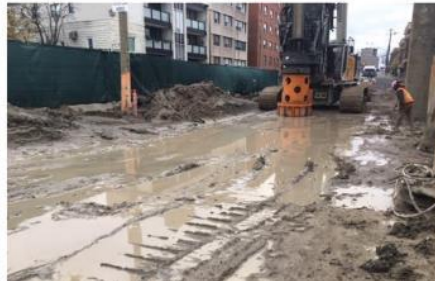
Fig 7: Example of a poorly prepared platform with poor drainage
