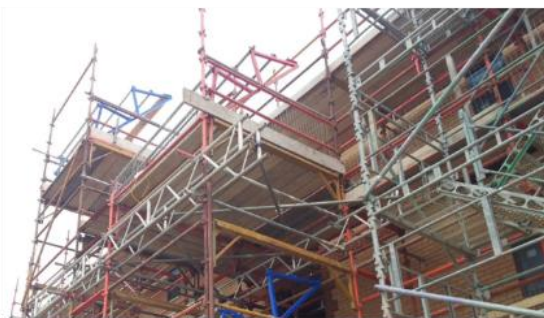
Independent access scaffolds with cantilevered spurred platform
