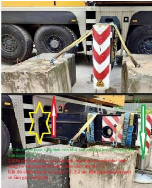
Photographs show concrete blocks and slings being used to hold down an extended crane outrigger
